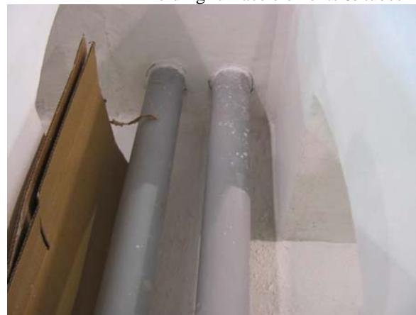
Holding furnace elements & tubes
